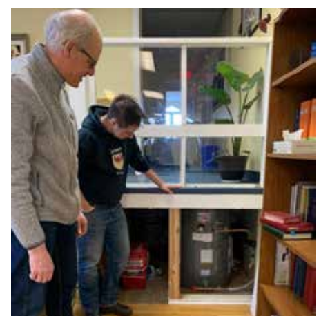
Parishioners Hans Posthuma and Charlie Scromeda check out the small hot water tank.
