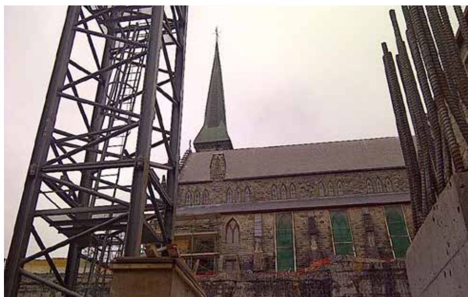
In 2013, the Cathedral's hall was gone and excavation for the first tower well underway. Staff received training for the next four years in patience and forbearance.
